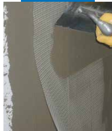
Smoothing insulating panels reinforced with a Fibreglass Mesh drowned into the coat of Mapetherm AR1
