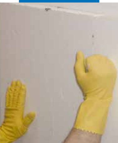
Applying pressure on the panels once they have been installed. This is to ensure a good bonding to the surface
